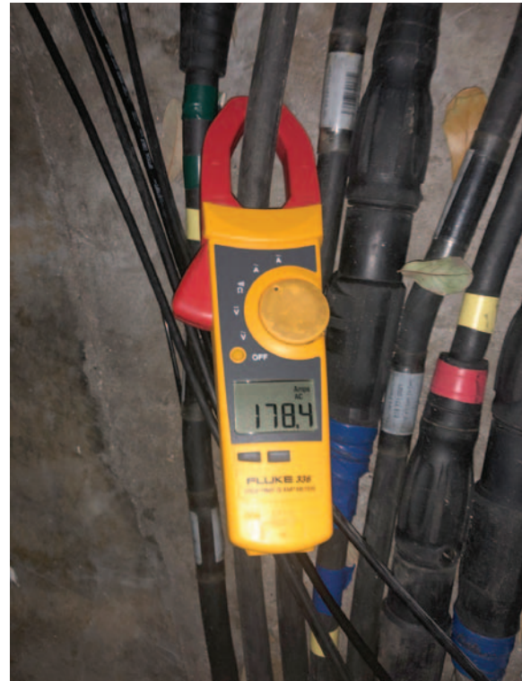
Clamp meter current reading corresponding to the FLIR infrared image in Figure 1.
