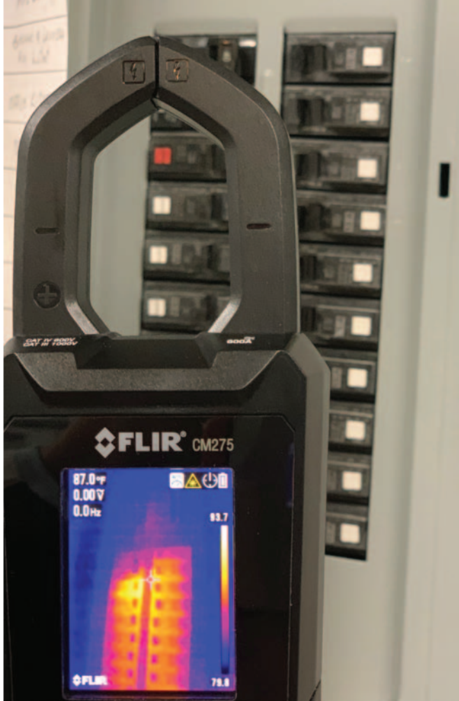
FLIR CM275 multimeter showing infrared camera monitoring breaker temperatures in an electrical panel.
