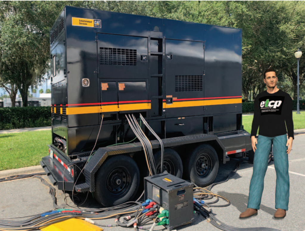
The availability of engine-generator sets like the MultiQuip SG1400C4F won't be limited by AB 1346—but they might be too big and expensive for small production.
